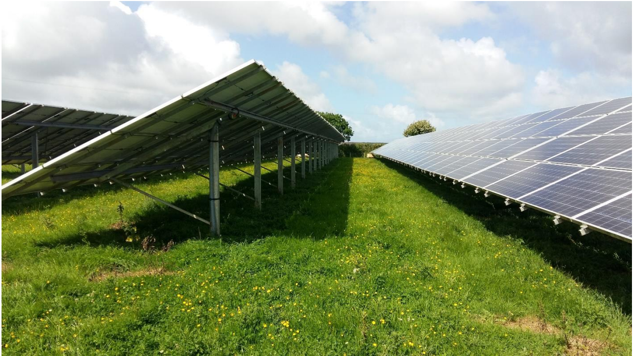
Image 3.1 Typical Solar Panel (image provided by RES)
