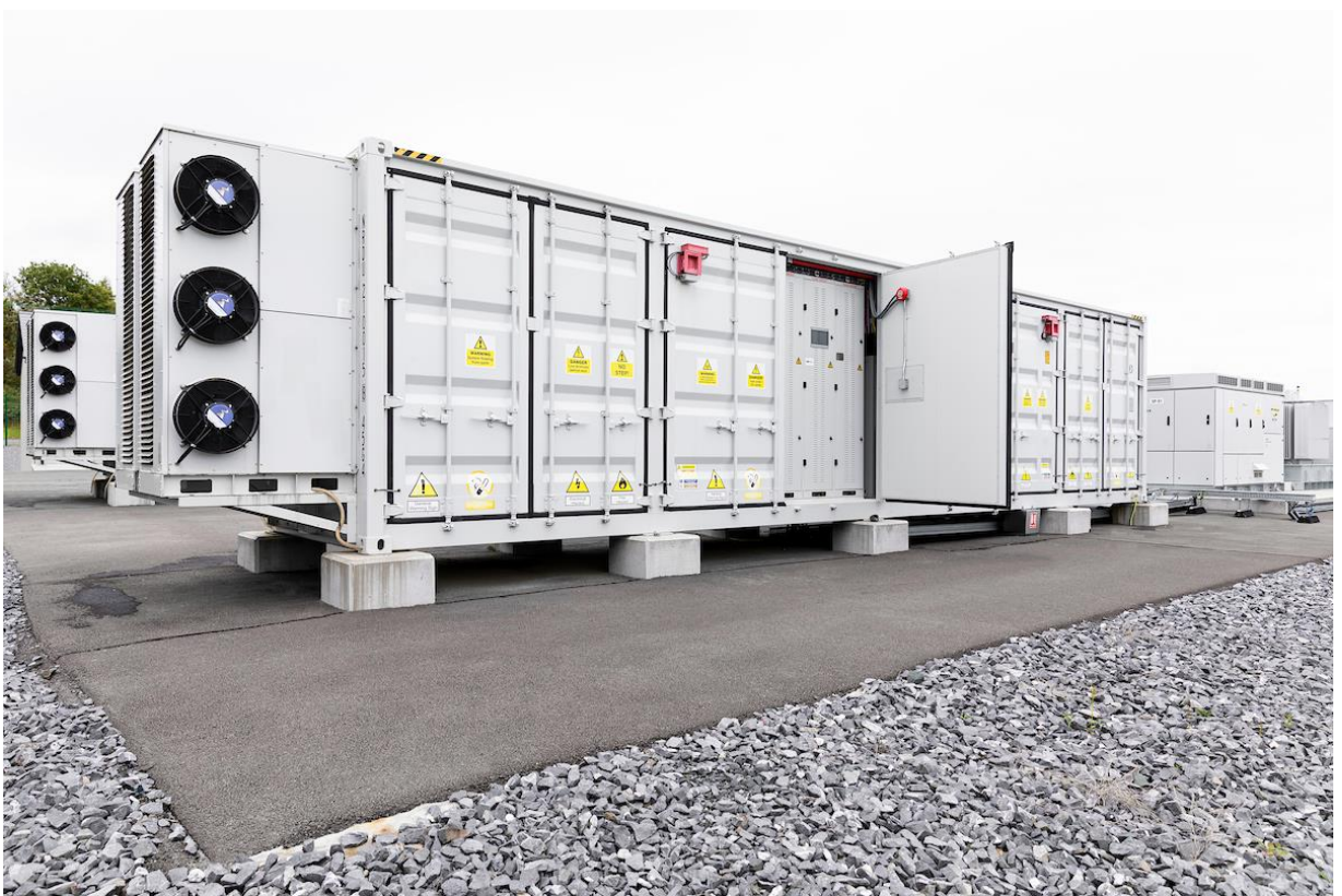
Image 3.2: Typical battery storage container (image supplied by RES) 5
